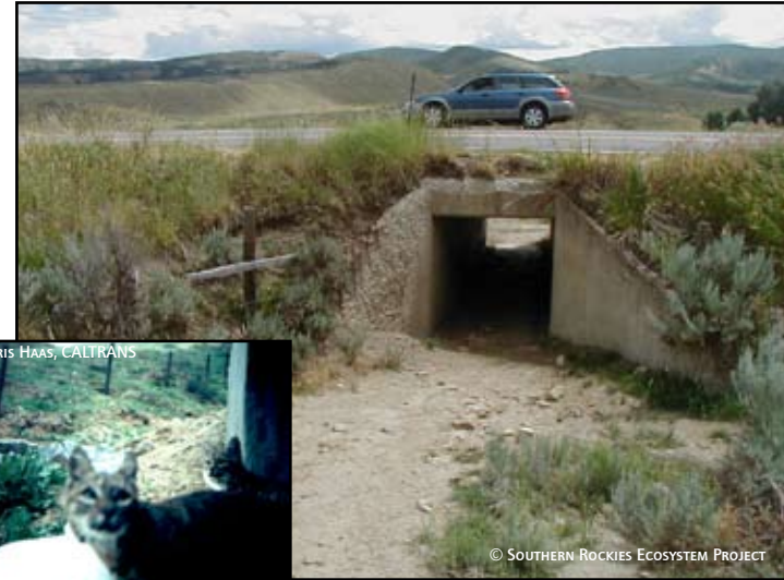
BOX CULVERT ON HWY 13 SOUTH OF CRAIG, COLORADO (ABOVE). BOBCAT USING A BOX CULVERT IN RIVERSIDE, CA UNDER CA 71 (LEFT).
